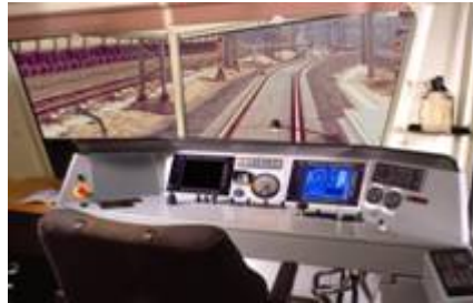
Train Control - Alcatel
