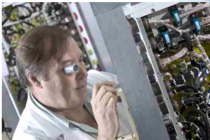
Working with the Electrical Load Management System (ELMS). This system is classed as Level B safety category in accordance with DO-178B standards.
